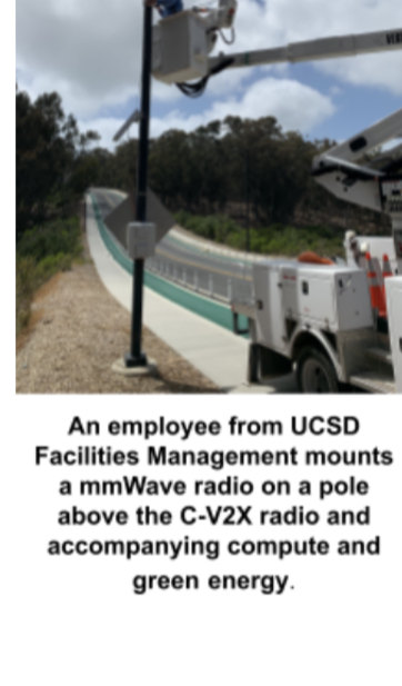
An employee from UCSD Facilities Management mounts a mmWave radio on a pole above the C-V2X radio and accompanying compute and green energy.
